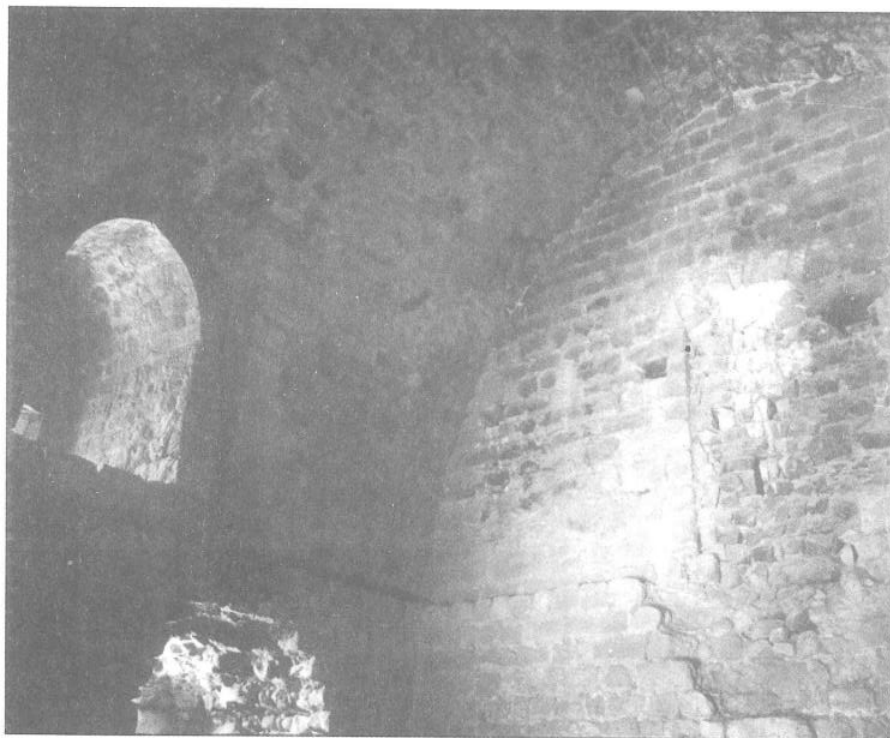
3. The ground floor room of the tower with blocked entrance and a loophole (looking west)
